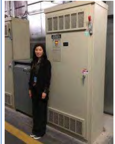
VFD Powering a 350 HP motor
